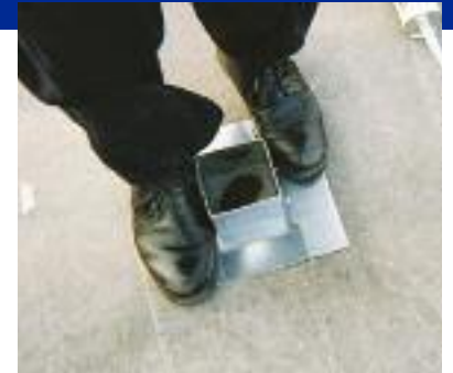
6) Apply pressure to activate MicroSealant adhesive. Run pipes, etc. Use excess tape or other to fill gap between pipe and roof before adding sealant. Go to Final Step #7.
