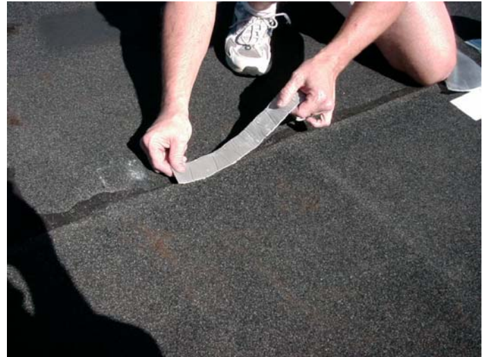
Figure 1: After sweeping repair area of debris, remove release liner from one side of EternaBond DoubleStick and apply to roof surface.
