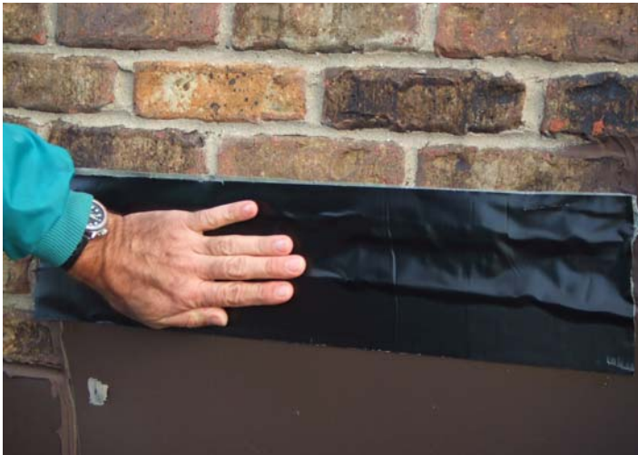
Figure 2: Apply EternaBond RoofSeal or RoofSeal-Plus bridging from wall surface to flashing tins or over termination bar to roof type (Modified, EPDM, TPO, Hypolan, etc.)
